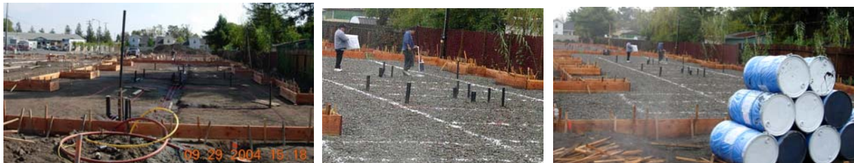
Left to right: Once the forms are up and the slab bases are rocked, chalk is used to lay out the location of the under-slab vents. Containers on right are the liquid used to seal the system.
