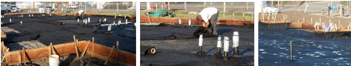
Left to right: Once the first layer has been checked thoroughly for leaks and sealed the top coat is then applied. The top coat is a rubberized fabric that is laid over the first coat exactly. All joints are carefully overlapped. Edges are folded up the concrete forms. Areas not covered will be exterior porches. Once all six buildings were prepared and checked, the slabs were ready to be cabled. The system is wrapped up the sides of the forms so that the perimeters will be sealed.
