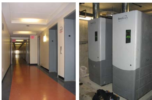
Energy efficient lighting and boilers
