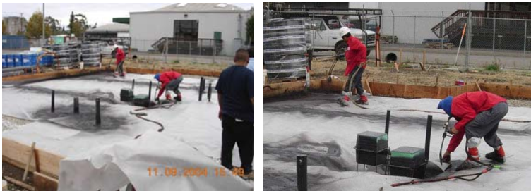
Left to right: Once layout is complete and all joints are sealed the first coat of fabric is placed over the assembly. The first coat of liquid boot is sprayed on. Each sprayer has two nozzles which hold two components that combined become a strong sealant.
