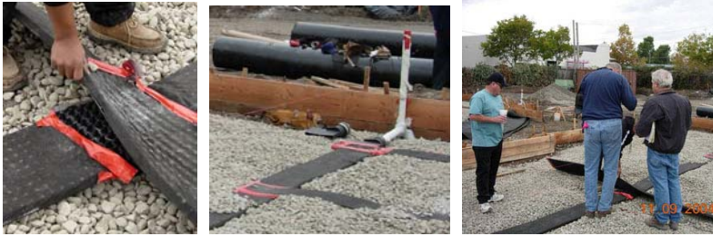
Left to right: Flat egg crate type vents are laid down over prepared rock and sealed at connections. Connections to pipes are at the perimeter. Any vapors that could percolate up from the soil will hit the rock layer which will be carefully sealed. These vapors then migrate sideways into the permeable vents. Once inside they will be drawn by the pipes by convection and out to the roof. All work is carefully inspected and documented.
