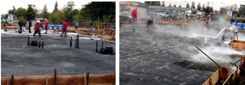
Left to right: The first layer is completely saturated and all joints are carefully sealed. Once this is complete a Smoke Test is done. The smoke test will detect any leaks in the system. Smoke is blown through a hole in the middle of the system and any leaks are promptly sprayed.
