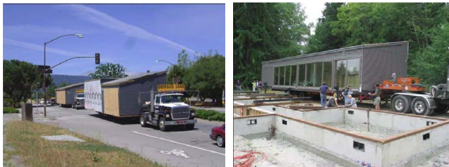
Modular Glidehouse being shipped to the site then lowered onto the foundation
