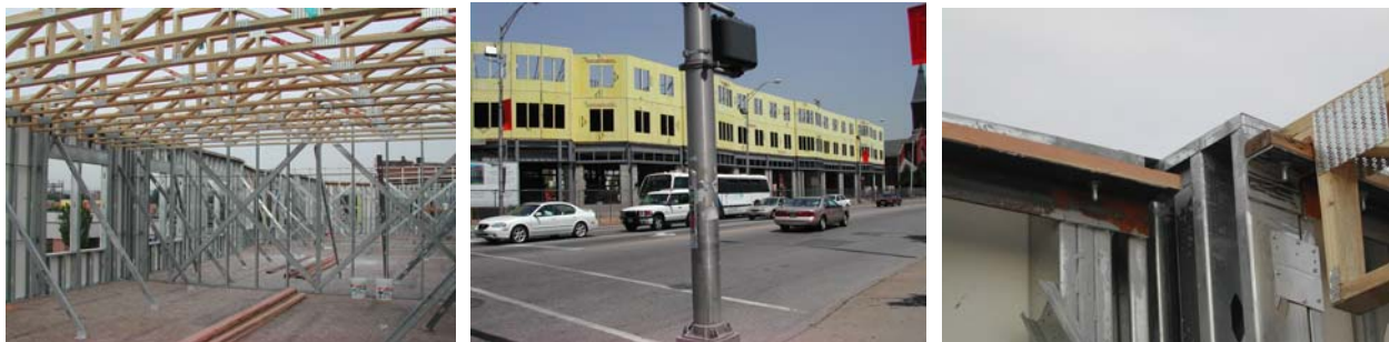
Left to right: Steel framing and wood trusses (Type 3 construction); two of four floors in place; panels fabricated with internal support angles which receive nailer for trusses which keeps trusses entirely out of non-combustible exterior wall assembly.
