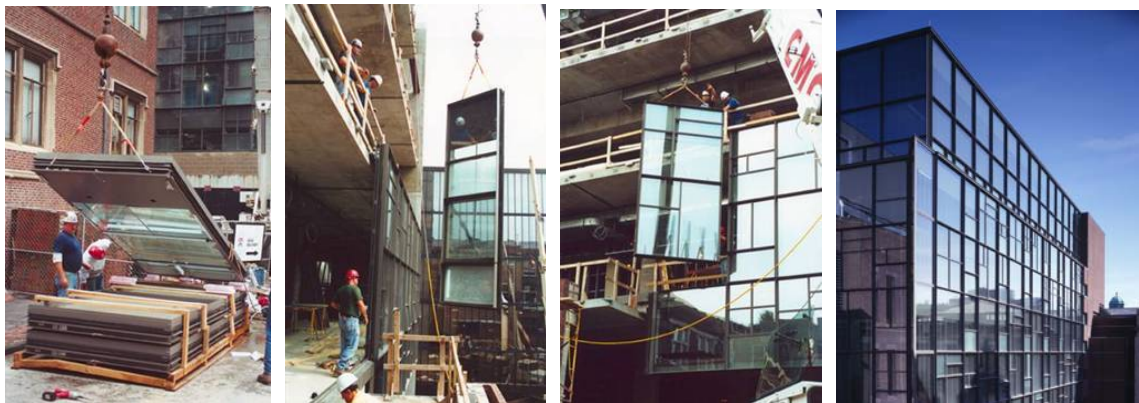
Melvin J. and Claire Levine Hall, University of Pennsylvania Left to right: Pre-fabricated curtainwall system being installed and the completed project
